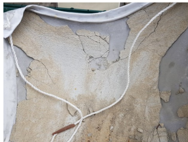
Figure 9. The result of an uneven surface across the flexible formwork caused cracking throughout the thin shell.
