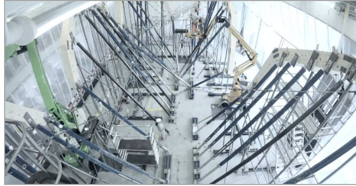
Figure 4. A portion of the required formwork for Philippe Block's HiLo shell roof, ETH Zurich
